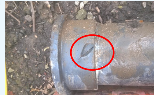
Source of the leak – a cracked 4" underground water pipe
